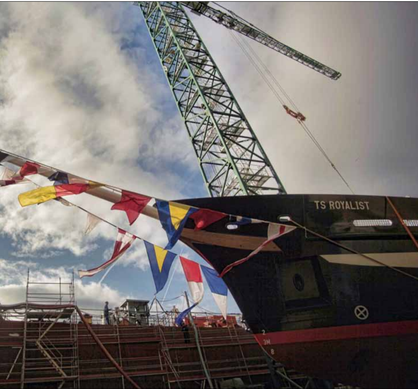
sits in the shadow of a Norwegian North Sea supply vessel under construction at Astilleros Gondán
