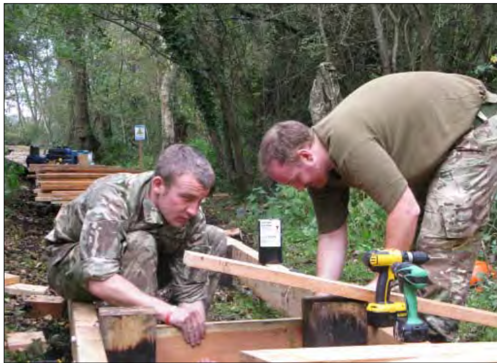
● LAET Gav Babb and LAET Shaun Cain form joists for the boardwalk
